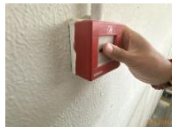
Fire alarm test is ok.JPG
